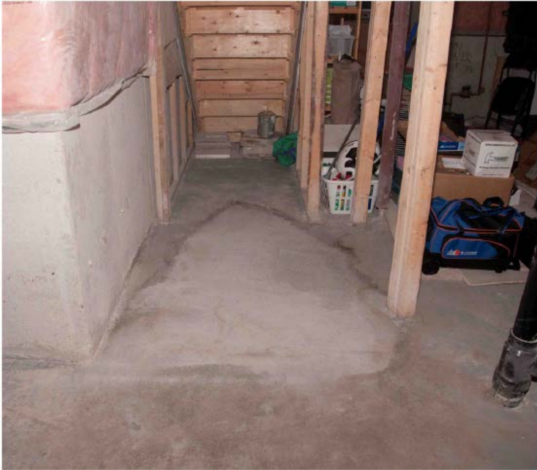
Fig. 5. Suspect location identified in basement of residence in Toronto, Canada due to area of different construction.
