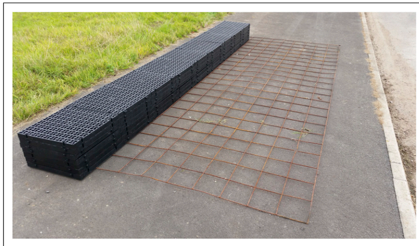
Figure 3. The data fusion testing mesh in-situ, with a simulated cover depth of 289 mm set up.
