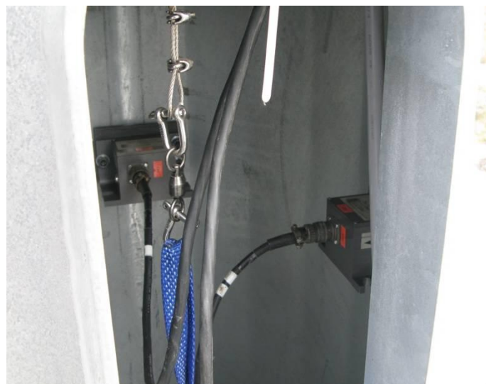
Figure 7 Two uniaxial CMG-5U accelerometers in situ inside the Proven 35-1.
