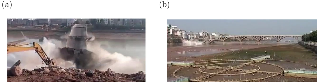
Figure 1: (a) The demolition of a bridge in Guangxi, China. The excavator in this picture was used to initiate a failure at one end of the bridge. The figure shows the resulting periodic failure process propagating through the structure, where the supporting columns fail sequentially. An alternative view of this process is presented in (b). (online version in colour)
