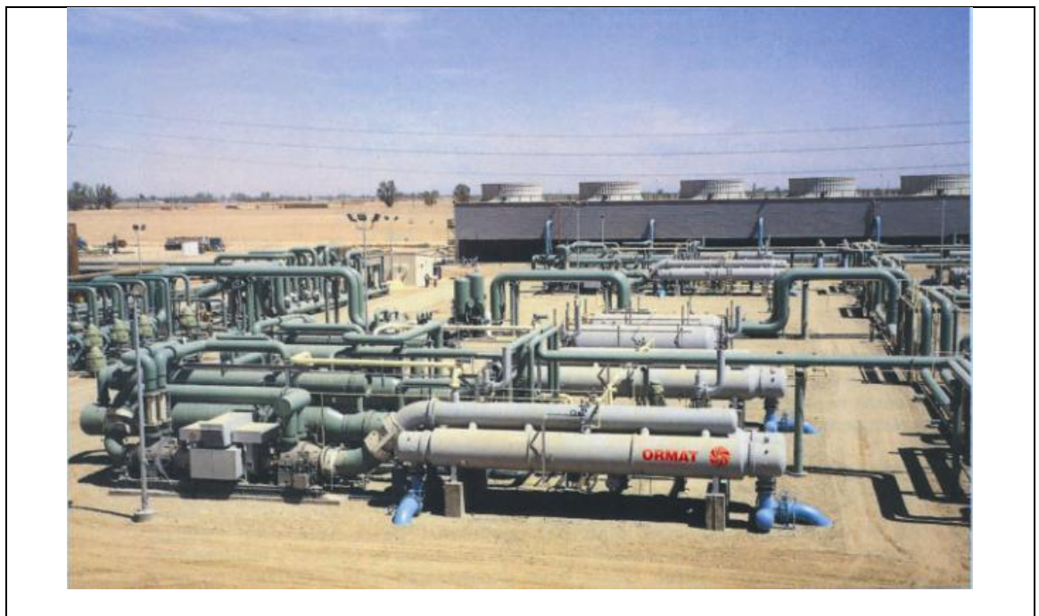
Figure 51: ORMAT ORC Geothermal System in Nevada, USA
