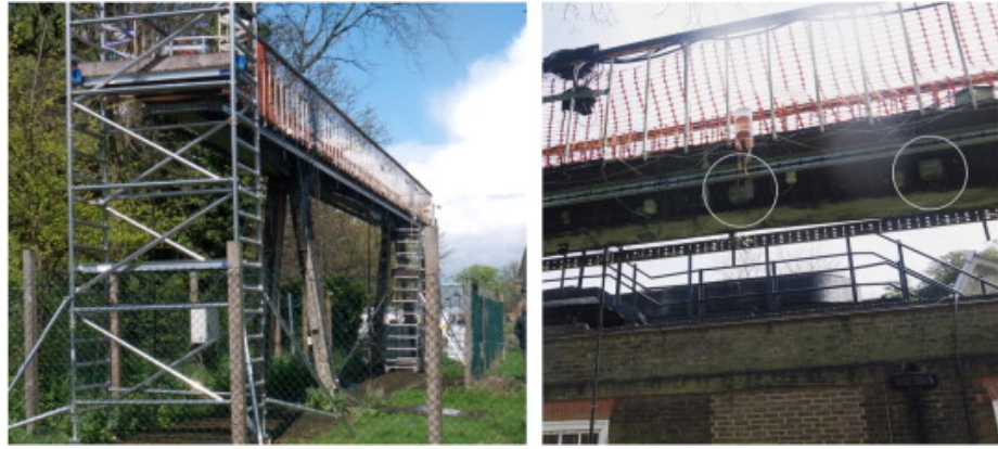
Figure 4.2: The NPL footbridge. The image on the left shows the bridge itself, while the image on the right shows two of the tilt sensors, which are circled in white (reproduced from Kromanis and Kripakaran [433]).
